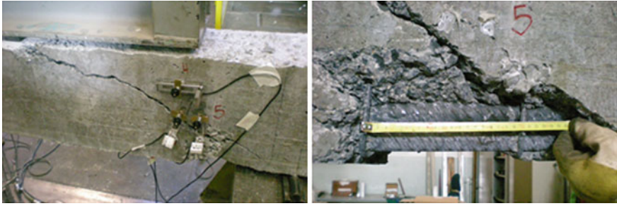
Fig. 4.16 Shear failure in B2 beams
